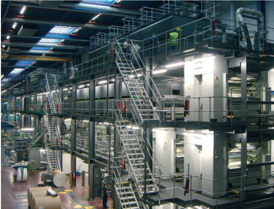
Roularta in Belgium recently installed the world's largest double-width newspaper heatset press — four COLORMAN towers each equipped with MEGTEC dryers to print up to 128 tabloid pages. Photo manroland.
